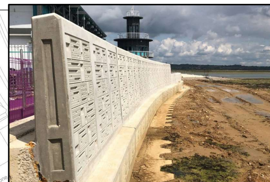
Opportunity to include ecological form liners to create textured surface on sea wall.
