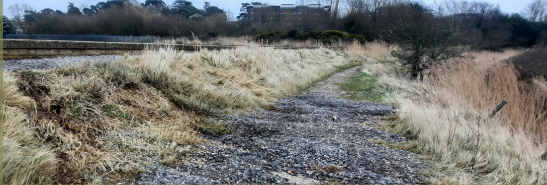
Damage to footpath and main embankment caused by Storm Barra
