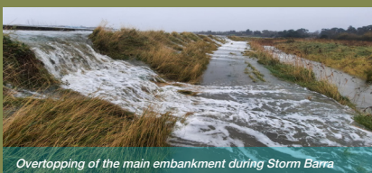
Overtopping of the main embankment during Storm Barra
