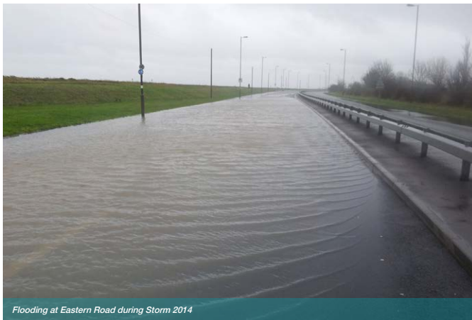
Flooding at Eastern Road during Storm 2014
