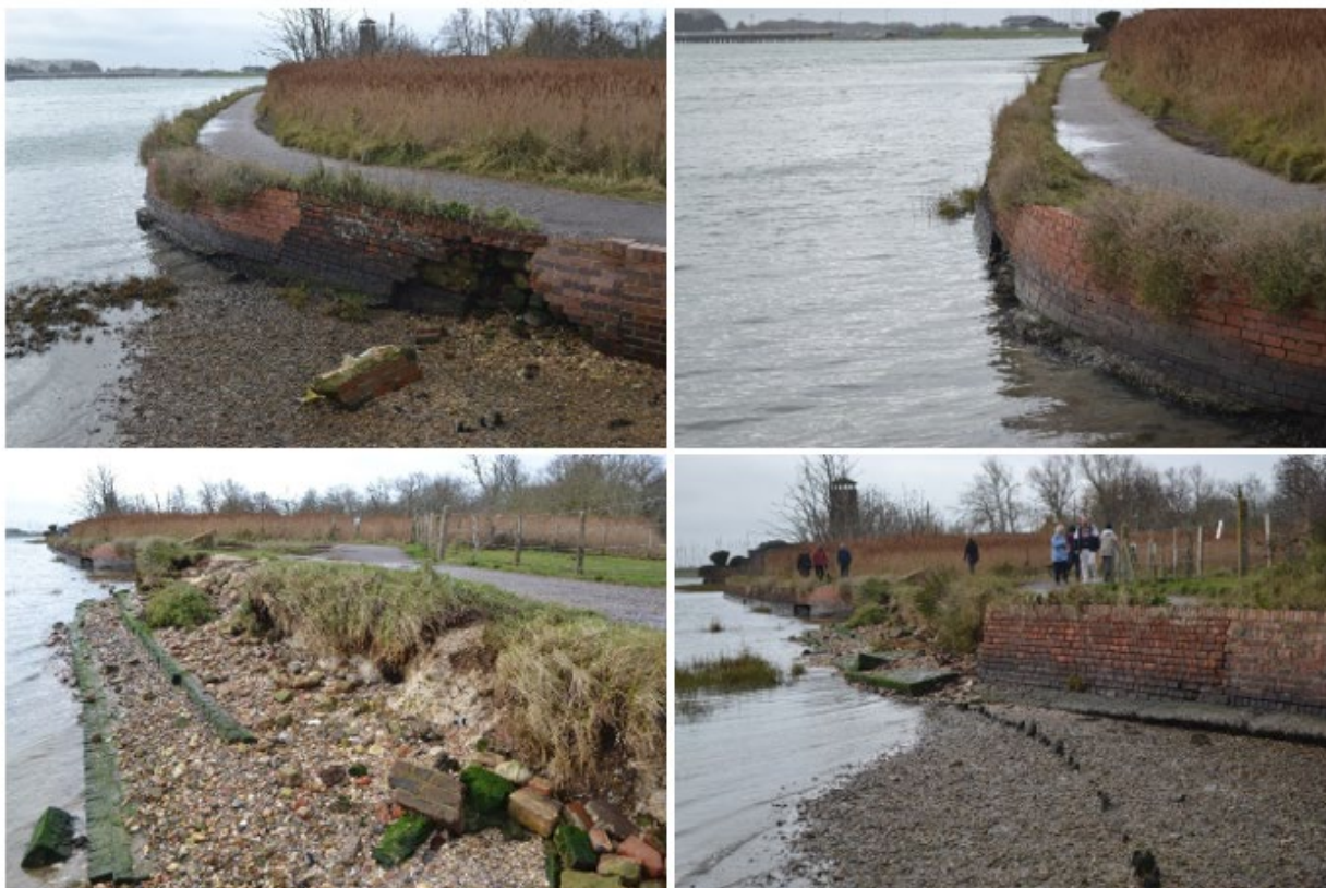
Figure 4 Damaged seawall at Langstone Mill. Photographs taken 4 th January 2023 (RHDHV 2023).
