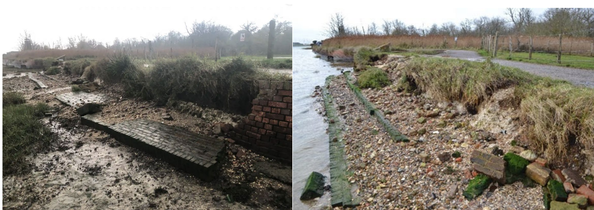
Figure 3 (Left) collapsed sea wall in spring 2022 (photograph coastal partners); (right) collapsed sea wall in January 2023 (photograph D. Brew, RHDHV 2023)
